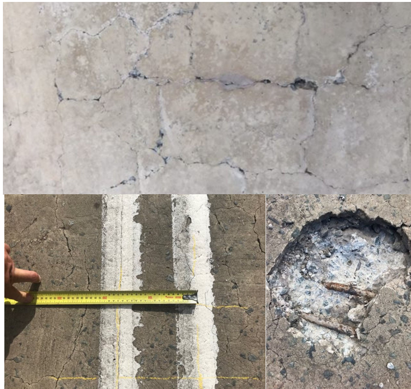
Figure 6 Bee Creek bridge deck slab deterioration
