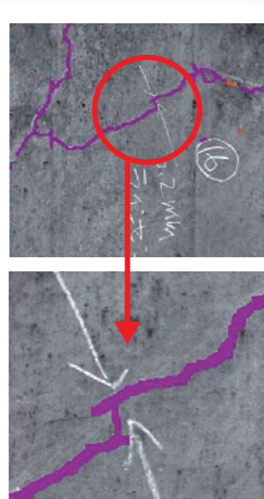
Crack analysis (minimum 0.2mm in width)
