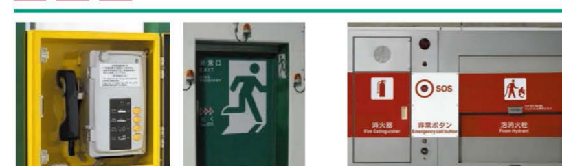
4 Emergency phone 5 Emergency exit 6 Fire extinguisher, foam fire hydrant, and pushbutton fire alarm
