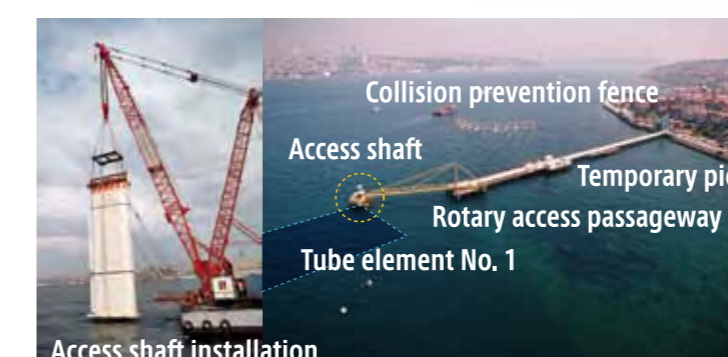
To reduce construction time, a prefabricated temporary "access shaft" was installed in the first immersed tunnel tube on the Asian side instead of in-situ construction of vertical shafts on both shores.
