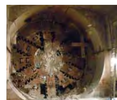
The moment of penetration The TBM seen from the inside of the immersed tube tunnel.
