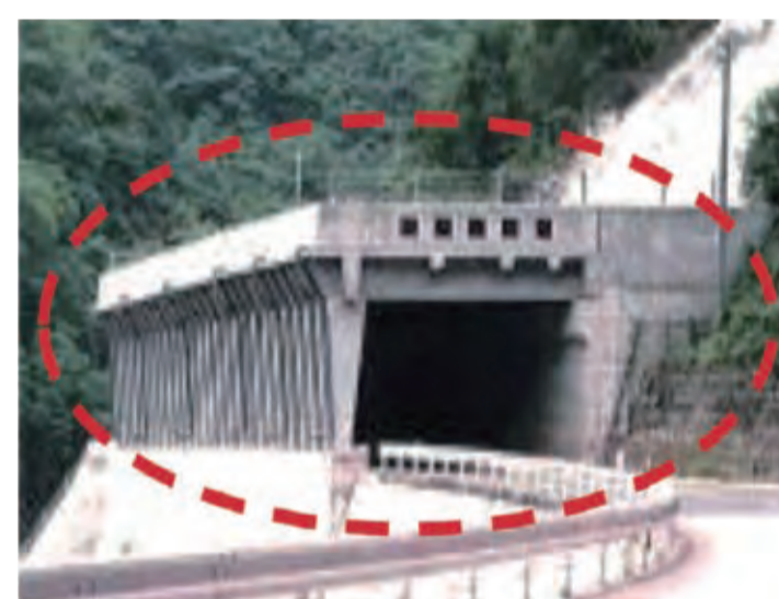
<Facility to protect against falling rock>
