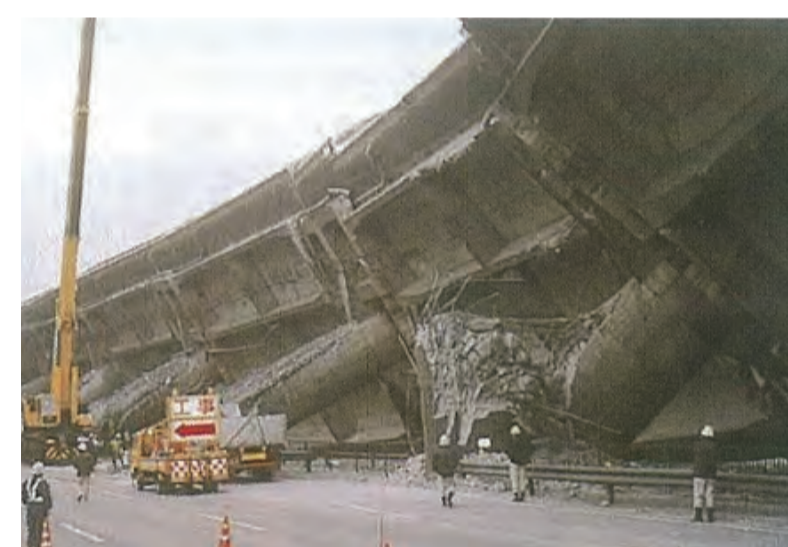
<Damage caused by the Great Hanshin, Awaji Earthquake in 1995>
