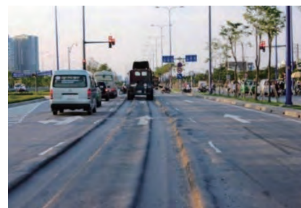
Examples of Damaged Road Pavement
