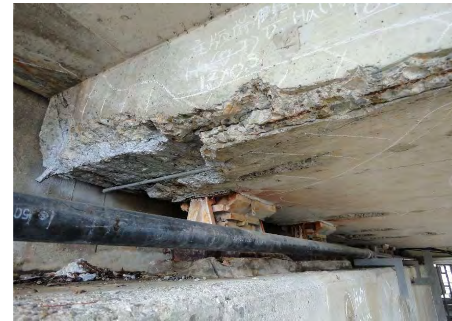
Concrete cracks and float
