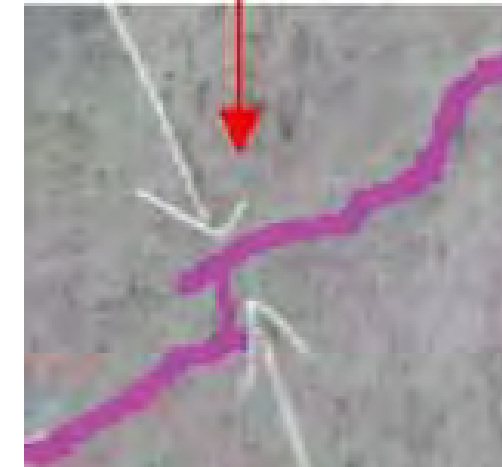
Crack analysis (minimum 0.2mm in width)
