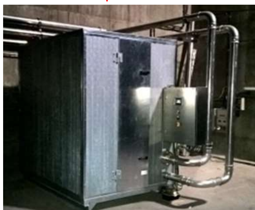
Plant room for dehumidification system
